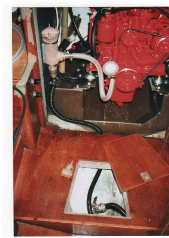
Figure 2 - Beta 20 Engine with Filter & Cooling Water Inlet (with Quarter Turn Ballvalve) The strainer was lowered later to bring up the static waterline.
