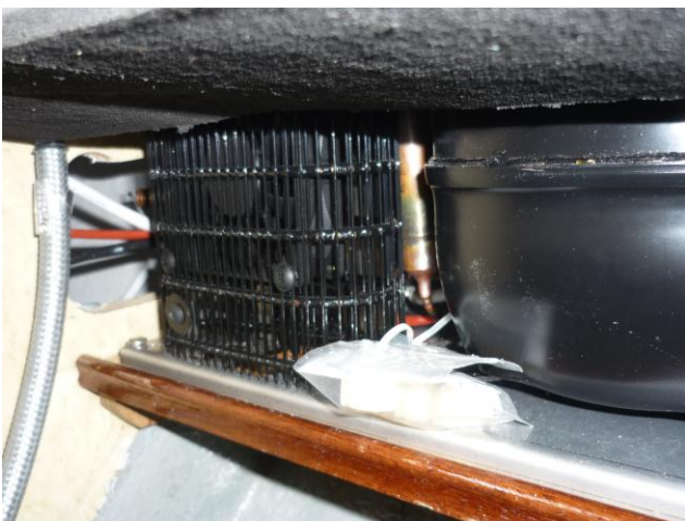
Compressor and heat exchanger in position behind the cooker with the “heat shield” swung up
